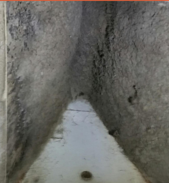
DIRTY EVAPORATOR COILS
